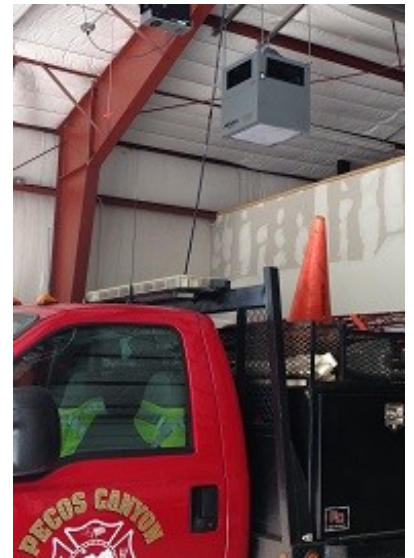
One of the three new exhaust fans which have been installed in the PCFR station.
